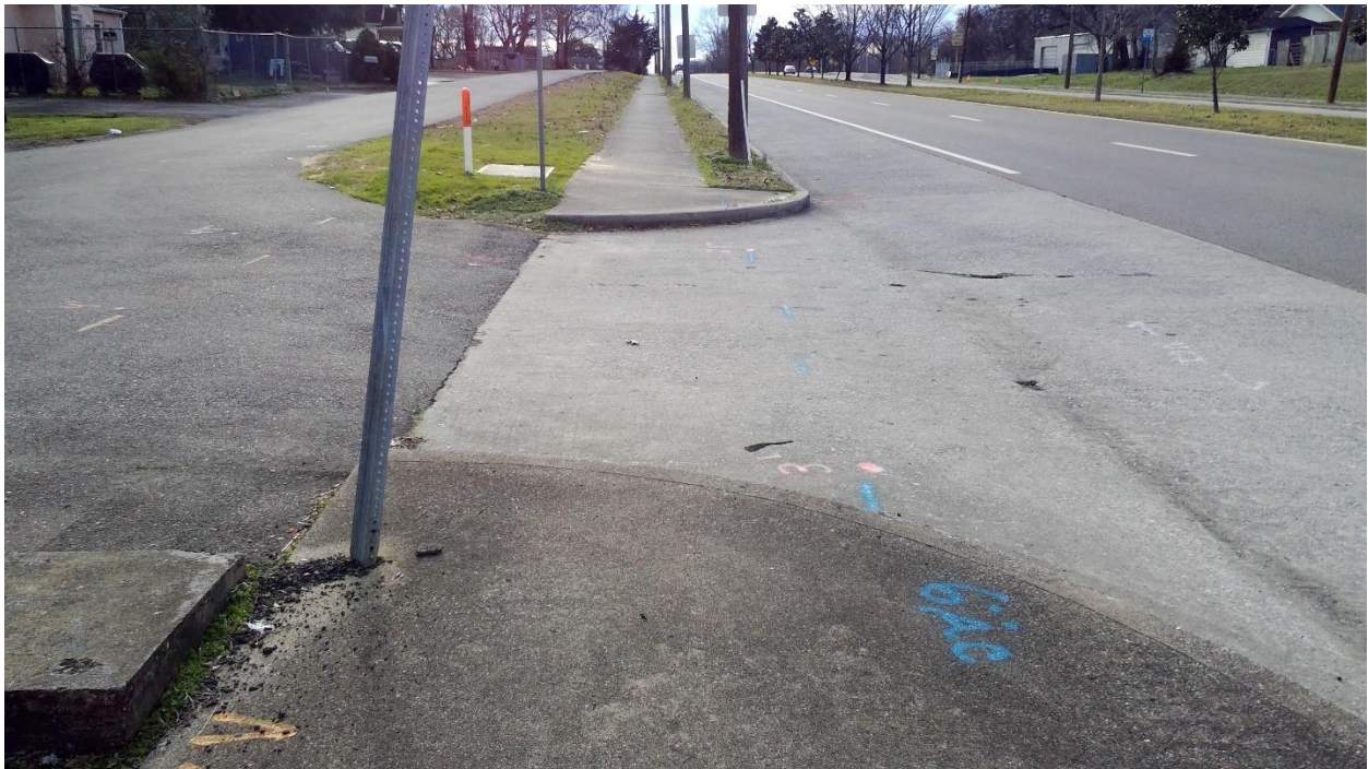
FIGURE 3: ASHEVILLE HIGHWAY (SR 168) AT SEAHORN AVENUE Demonstrates no curb ramps
