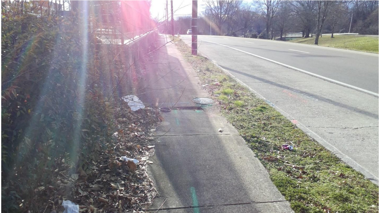
FIGURE 6: ASHEVILLE HIGHWAY (SR 168) Demonstrates deficient sidewalk condition and obstruction
