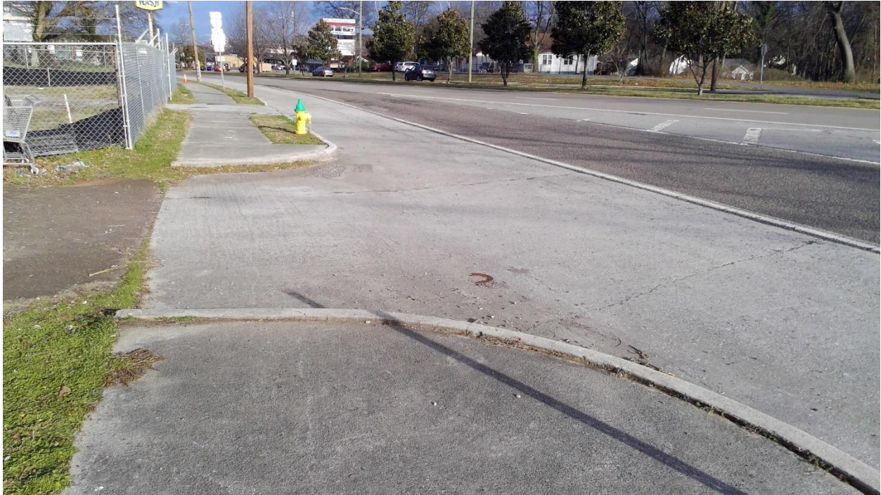
FIGURE 14: MAGNOLIA AVENUE (SR 1) Demonstrates missing curb ramps
