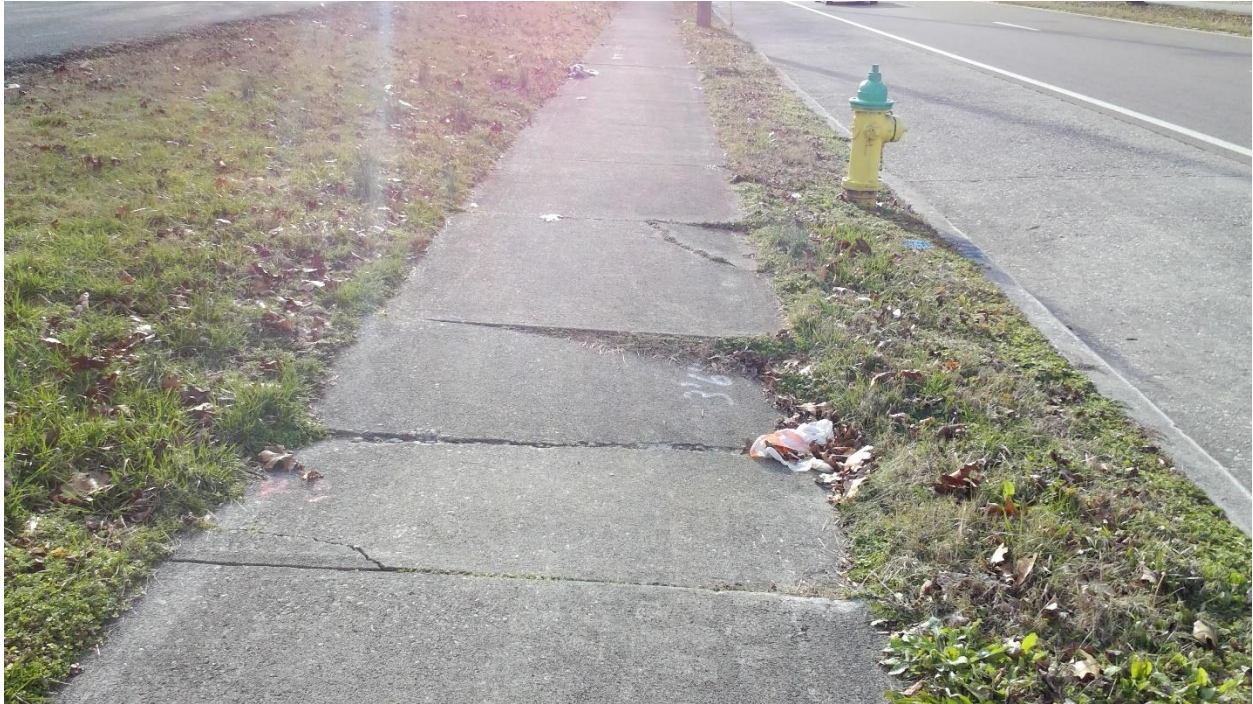
FIGURE 4: ASHEVILLE HIGHWAY (SR 168) AT SEAHORN AVENUE Demonstrates deficient sidewalk condition
