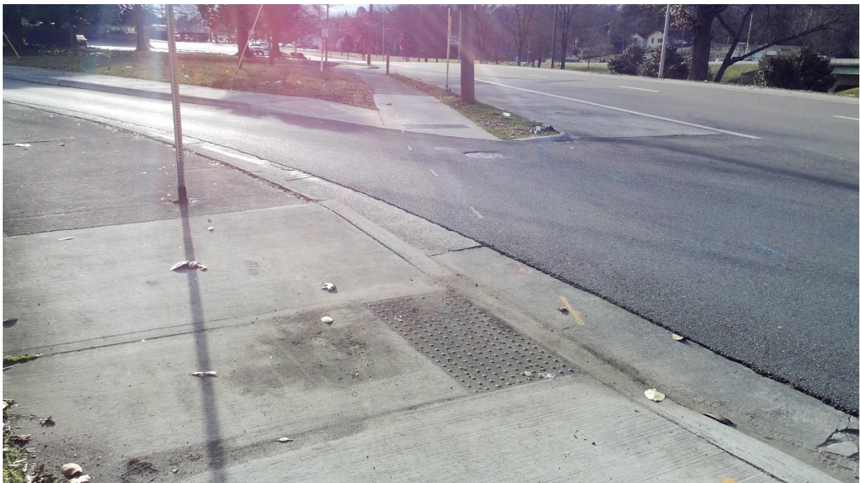
FIGURE 7: ASHEVILLE HIGHWAY (SR 168) AT MARTIN LUTHER KING JR. AVENUE Demonstrates curb ramps
