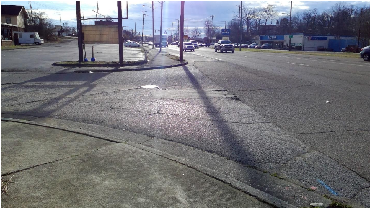
FIGURE 9: MAGNOLIA AVENUE (SR 1) AT SHELBY STREET Demonstrates no curb ramps
