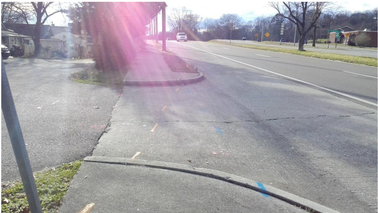
FIGURE 5: ASHEVILLE HIGHWAY (SR 168) AT SEAHORN AVENUE Demonstrates no curb ramps
